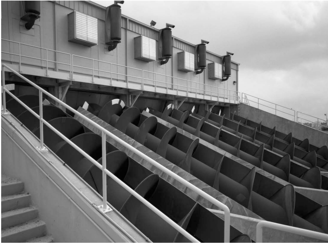
Enhanced versions of the Archimedean screw can lift 125,000 gallons of water per minute over an 11-foot barrier.
